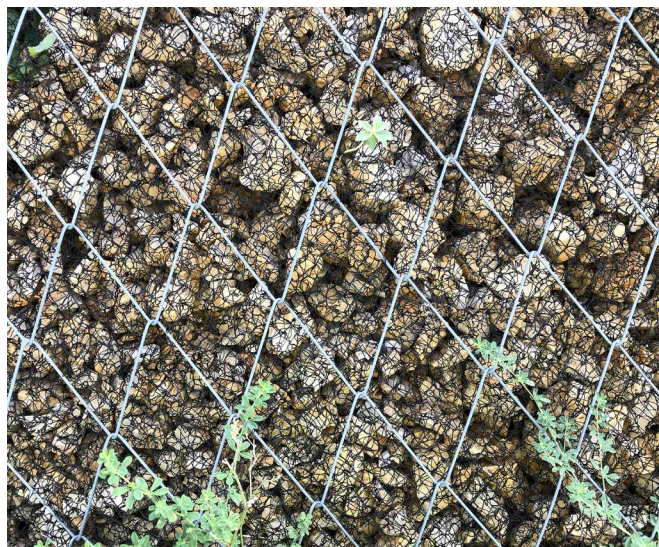
(fig. 8) Situation steep slope after five years (2020)
